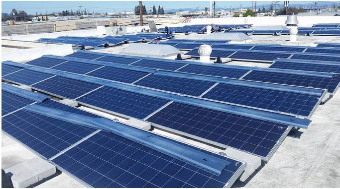
New 43 kW solar panel array installed on top of Toole's Garage
