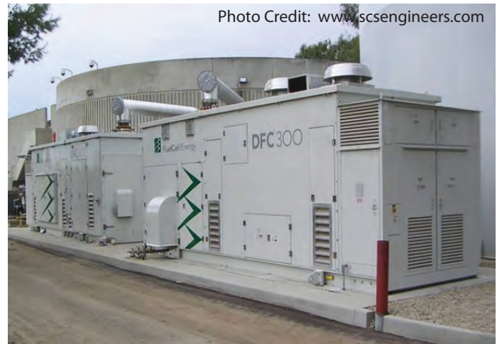
The City of Santa Barbara installed a cogeneration engine to convert excess heat into energy and uses it to operate the El Estero Water Treatment Plant.
